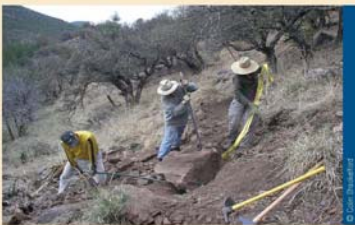
Many hands helped make this trail project possible. More than 1,800 volunteer hours went into the construction of this trail. If you would like to be a Nature Conservancy volunteer, please call our Fort Davis office at (432) 426-2390.
