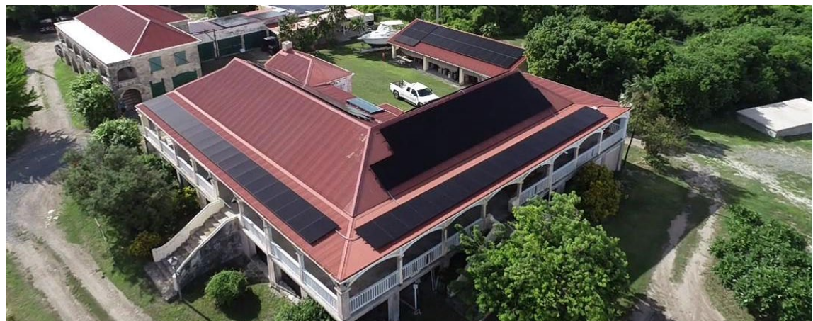
The installation of 164 new solar panels to power The Nature Conservancy's Coral Innovation Hub at Estate Little Princess marks significant progress towards achieving our 2030 goal of reduced climate impact for a livable world. Photo: © Matthew Davies/TNC
