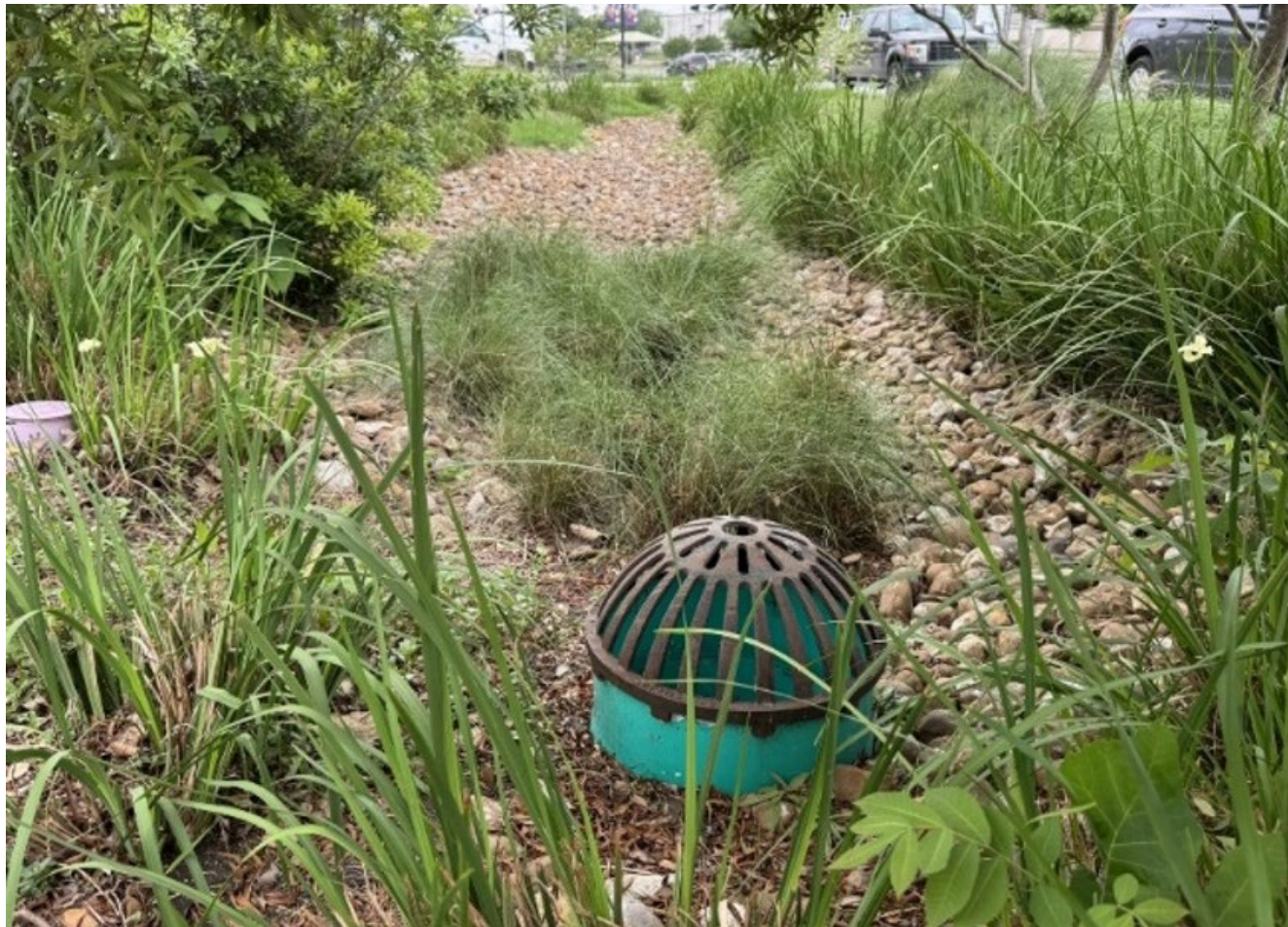
Figure 11-4. Stormwater overflow structure with domed debris grate
