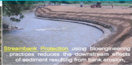
Streambank Protection using bioengineering practices reduces the downstream effects of sediment resulting from bank erosion.
