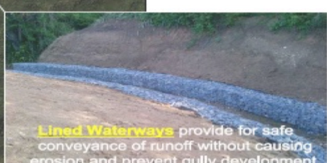
Lined Waterways provide for safe conveyance of runoff without causing erosion and prevent gully development.
