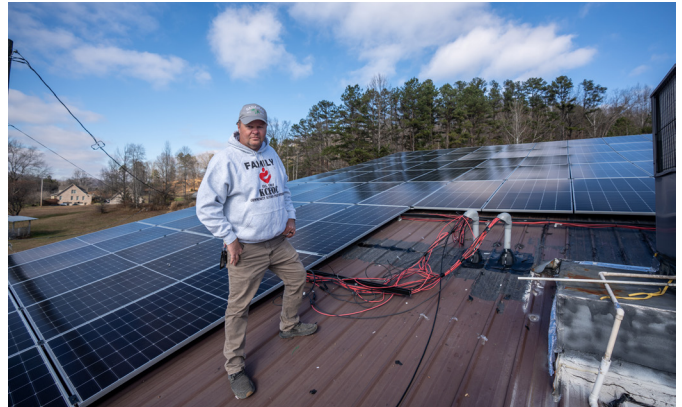
From top: Rooftop solar added in 2025 at Red Bird Mission in eastern Kentucky, reducing energy use so more funding can go toward community programs.; Solar panels installed in 2025 at the KCEOC Community Action Partnership facility in eastern Kentucky, helping lower energy costs and support local services. © Mike Wilkinson/TNC (both)
