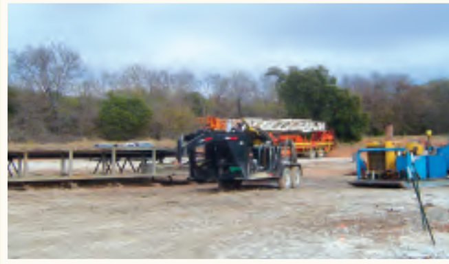
Construction of a typical pad site in the Barnett Shale © David Bezanson/TNC
