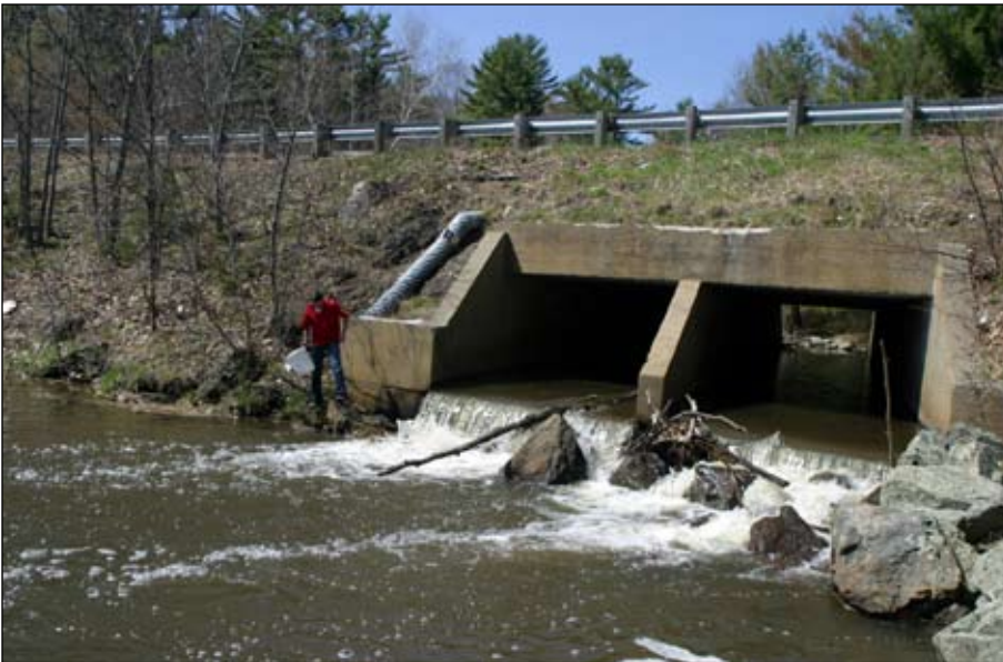
Even at high tide, migrating fish cannot climb this perched culvert to reach upstream habitat, leaving eels, herring, shad and other species without access to miles of good habitat. Nature Conservancy scientists like Ray Konisky (above) and others are looking at efficient ways to re-connect fragmented tidal streams like this one in Dover. Photo © Eric Aldrich / TNC
