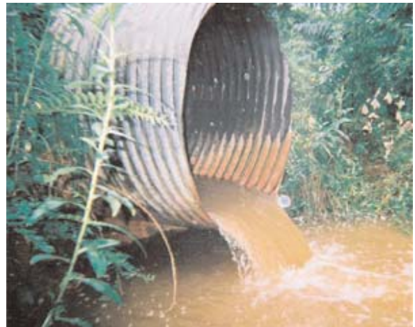
A culvert high above the water's surface makes it impossible for fish to swim upstream.
