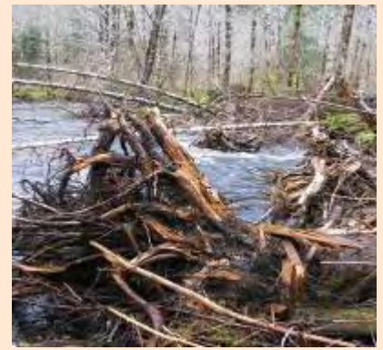
These root wads were placed in the stream channel to stabilize the stream bank and improve fish habitat. Photo: USFS
