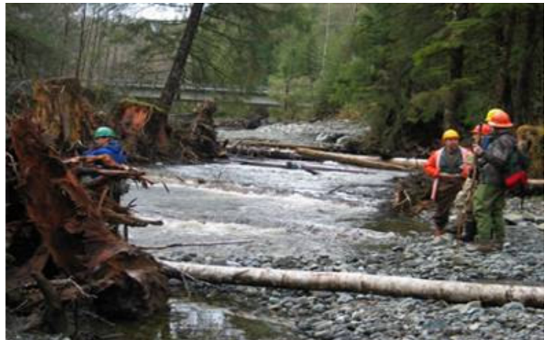
Adding woody debris to Fubar Creek stabilizes stream banks and improves fish habitat. © K Koski/TNC
