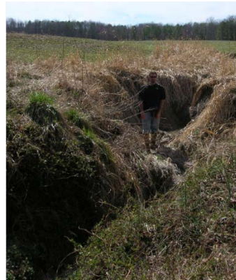
Erosion prior to restoration. 2005.
