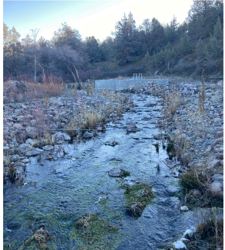
Figure 1. The new diversion structure looking up the reprofiled channel with riparian plantings
